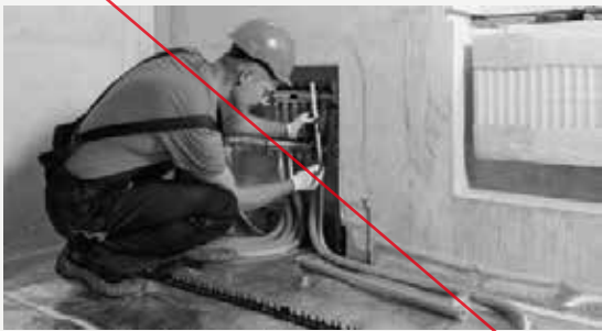
Laying pipelines Wasting Time, Labor, Money
